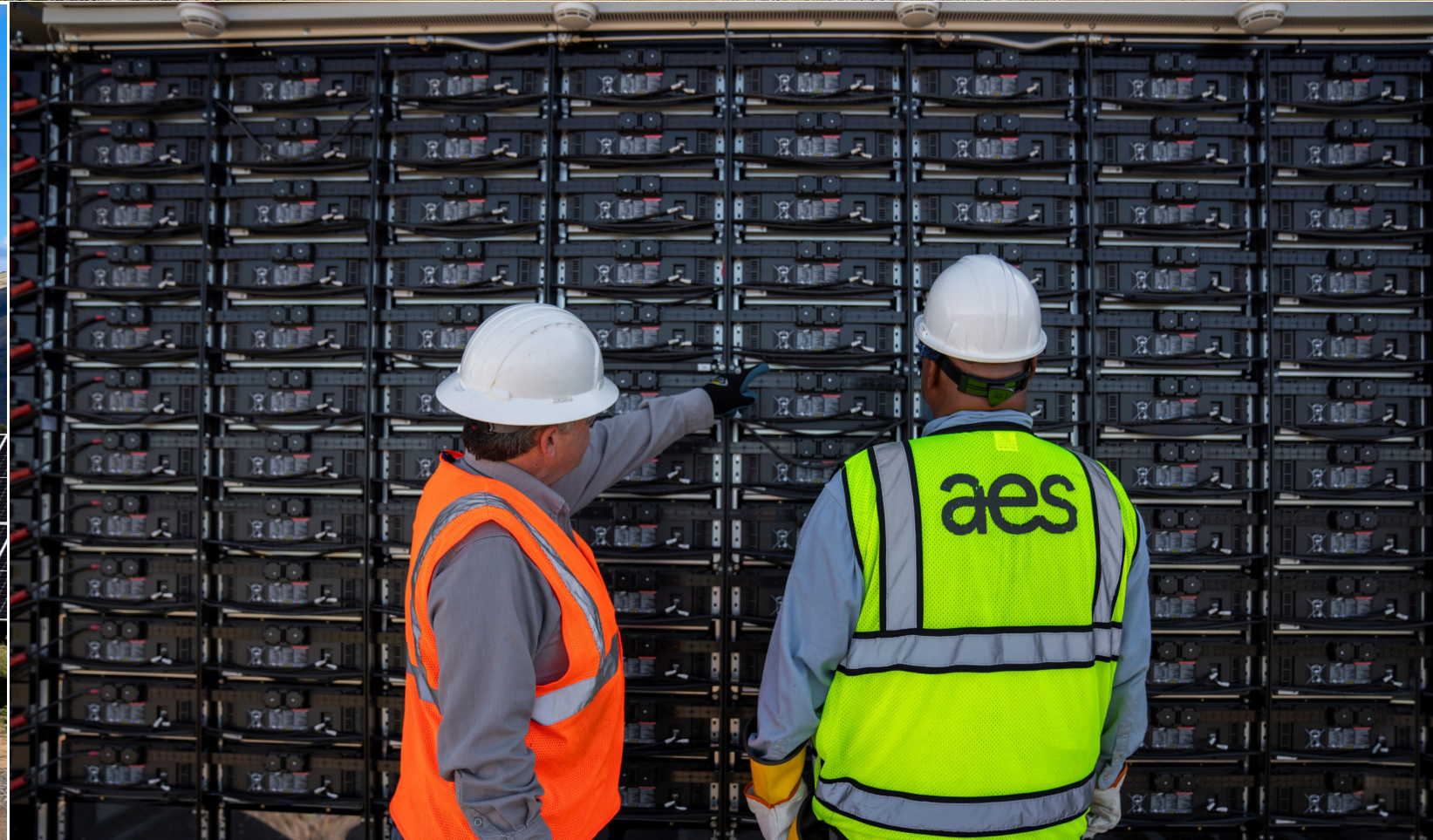
Battery Energy Storage System
