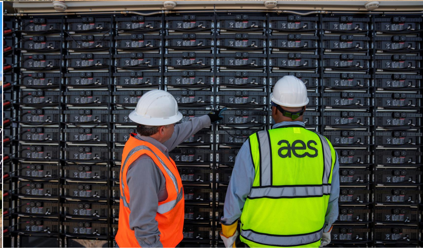
Battery Energy Storage System
